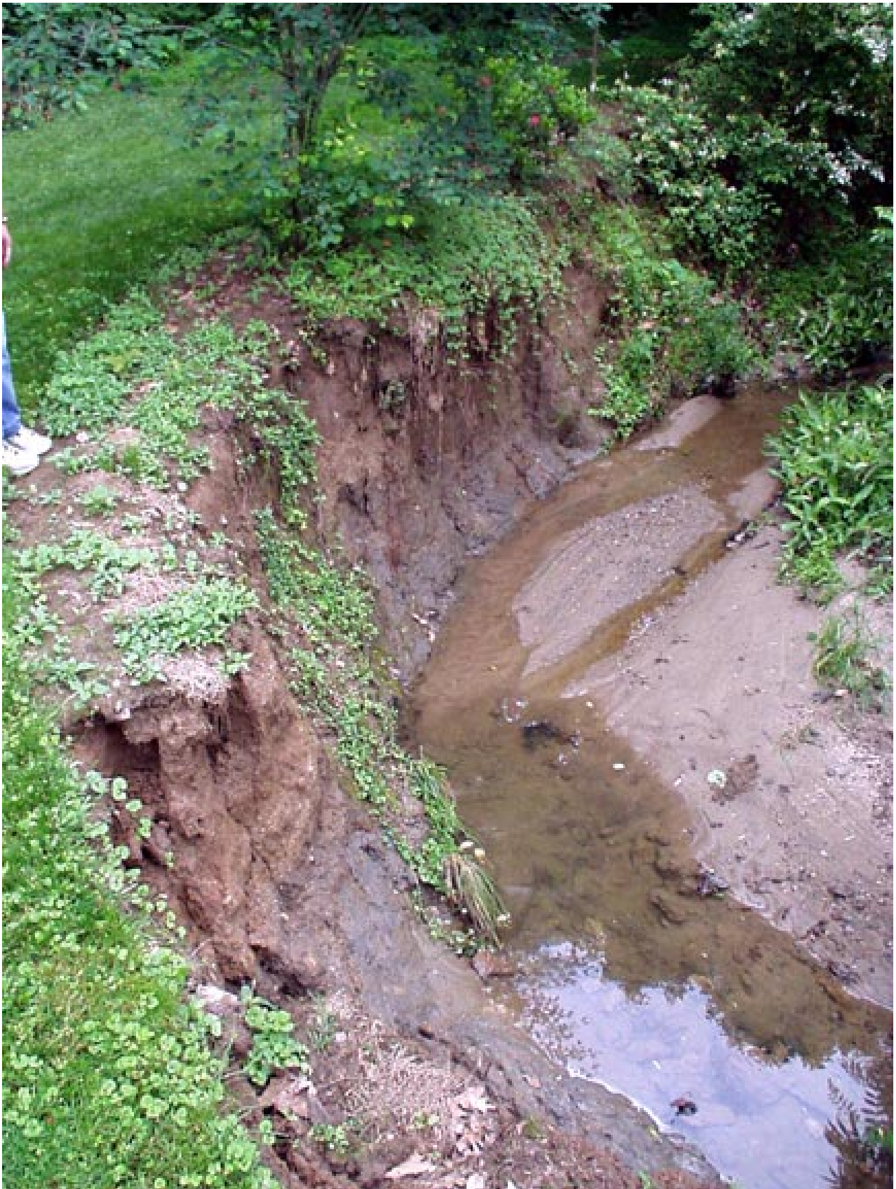
Figure 1 Erosion Along the bank of the Druid Hills High School Stream near Candler Lake.
