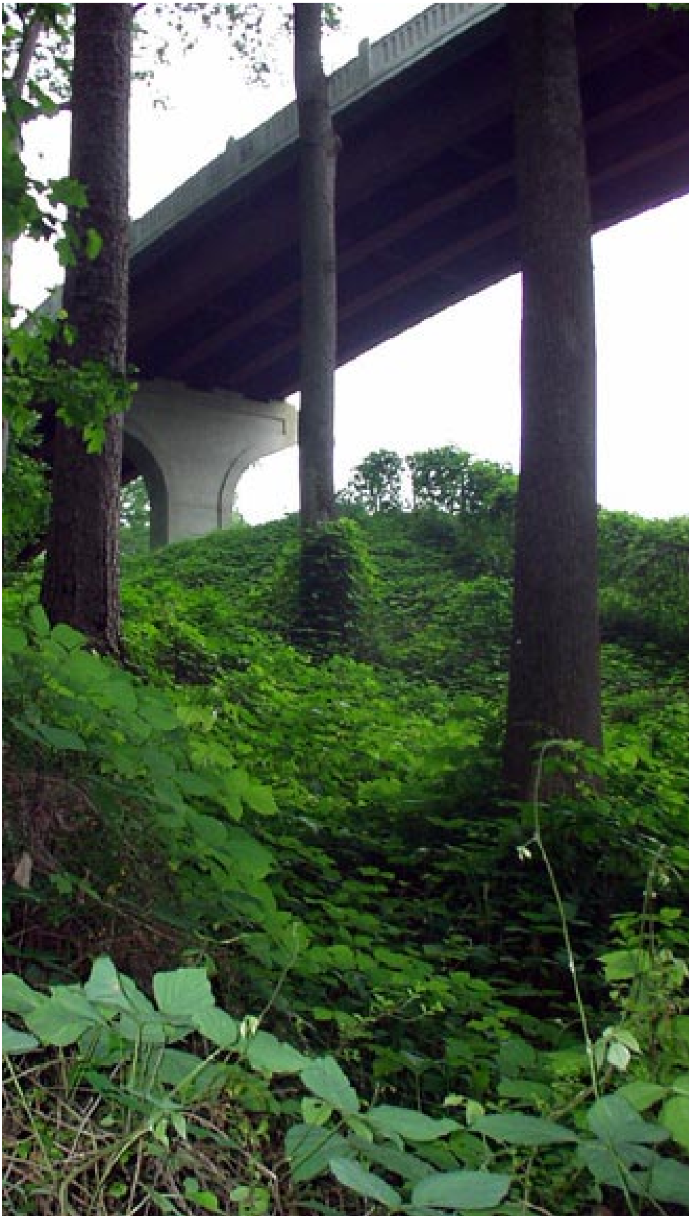
Figure 9 Kudzu is invading Lullwater by Starvine Way bridge.
