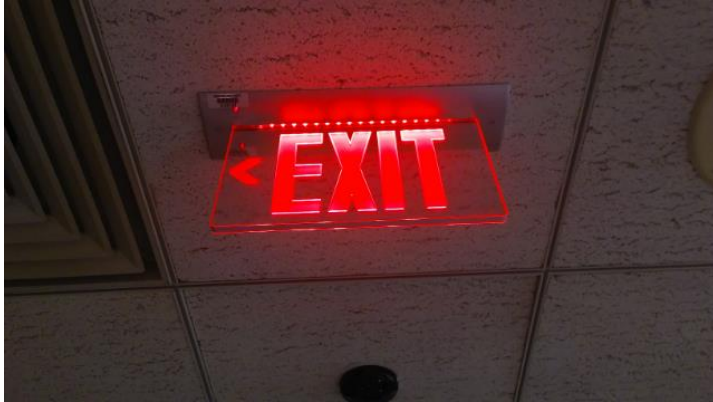
LED Exit signs installed in Emory University Hospitals
