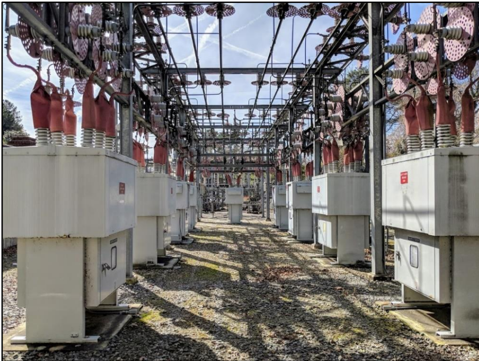
Emory Atlanta campus Oxford Rd Electric Substation
